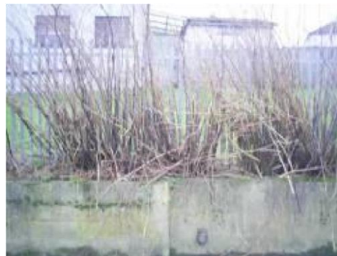
Fig 9. Reach 3: Japanese knotweed over mass concrete artificial bank.
